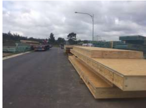
On site ready for install
