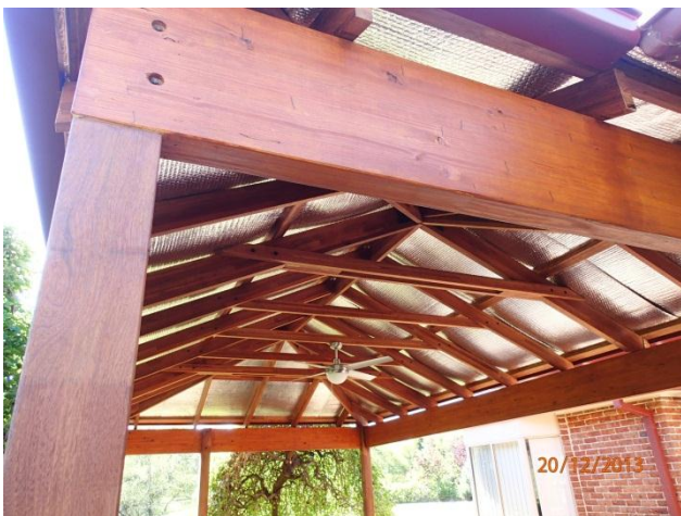
7.7m span Pitching Beam (on right)
