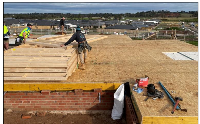
Pre-fab wall frame install starts as the sub-floor cassettes get the finishing touches.
