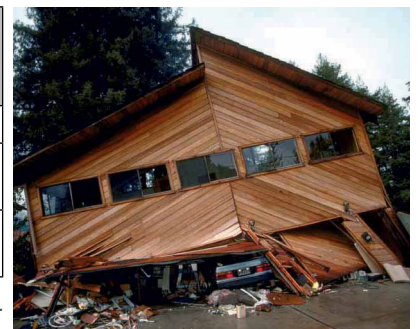
Fig 1 (above) Conflicting challenges of owners and designers. Fig 2 (right) An example of a failure due to lack of bracing.
